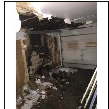
Above: The interior of the garage showing severe deterioration and mold issues. 09/12/2019
